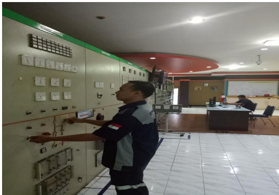
Lampiran 2 : Panel Control Mesin
