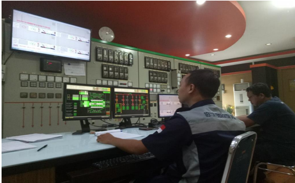
Lampiran 1 : Control Room Mesin
