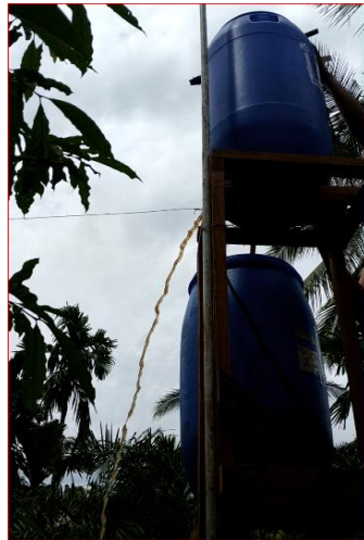
Back Wash Bak 1
